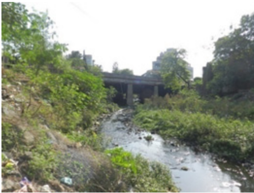
Dumping in Ram Nadi Channel
