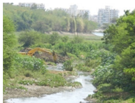
Silt deposition near Pashan Lake
